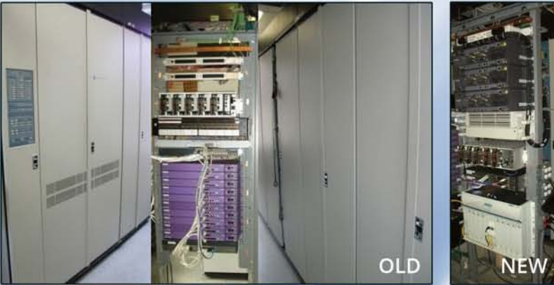
The old Siemens Switch, decommissioned (left) The new Metaswitch with Voice Mail and Caller ID (right)
