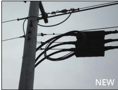
Fiber Optic Connection
