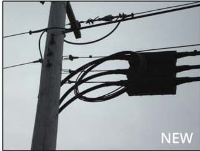
Fiber Optic Connection
