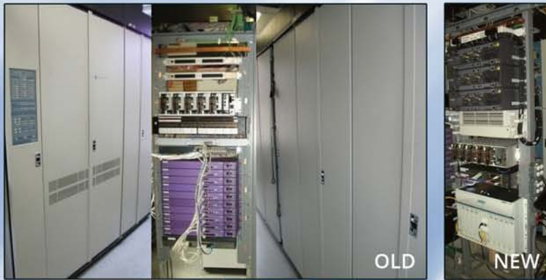
The old Siemens Switch, decommissioned (left) The new Metaswitch with Voice Mail and Caller ID (right)
